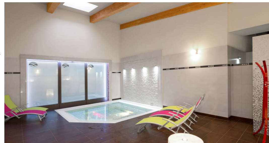
Saunas themselves do not need high illuminance levels. But it is important to use luminaires with a high protection rating – at least IP 44 for dry saunas, and IP 68 for steam saunas – that can resist high sauna temperatures.
